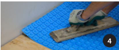
4 Unroll the membrane onto the thinset mortar and apply uniform pressure with a wood trowel.
