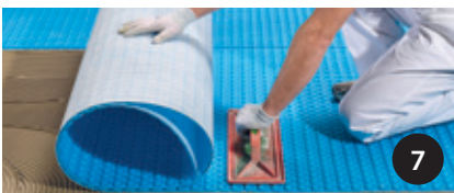
7 Lay the next sheets of membrane without overlapping and align square studs. Repeat previous steps until completion.
