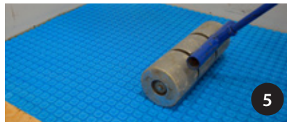
5 Use a 75 lb roller to achieve 100% thinset mortar transfer to the membrane.
