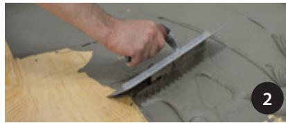
2 Key in the appropriate thinset mortar to the subfloor using the flat side of a trowel.
